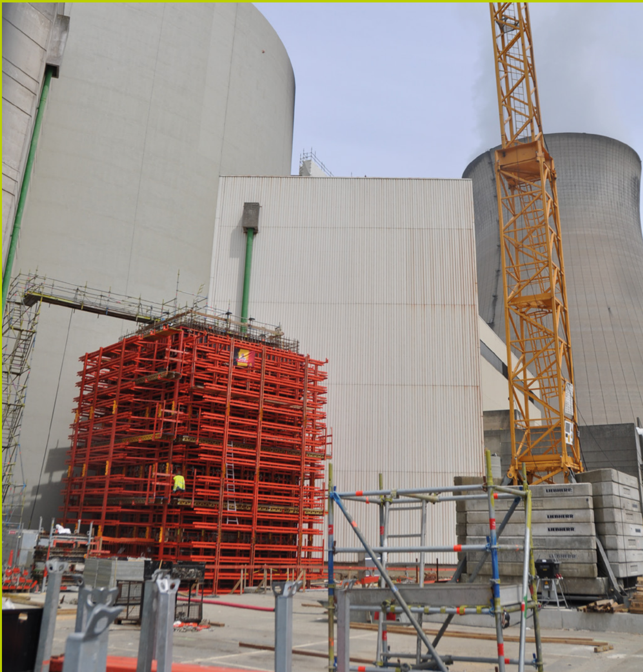
Installatie filtered containment venting-systemen.
